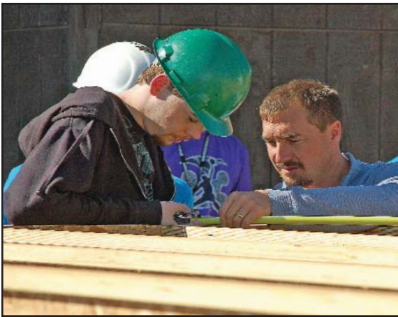
In the photo at the left, SBHS geometry-in-construction teacher Steve Lensegrav helps senior Todd Michaels measure the floor of the house currently being built at the high school.
